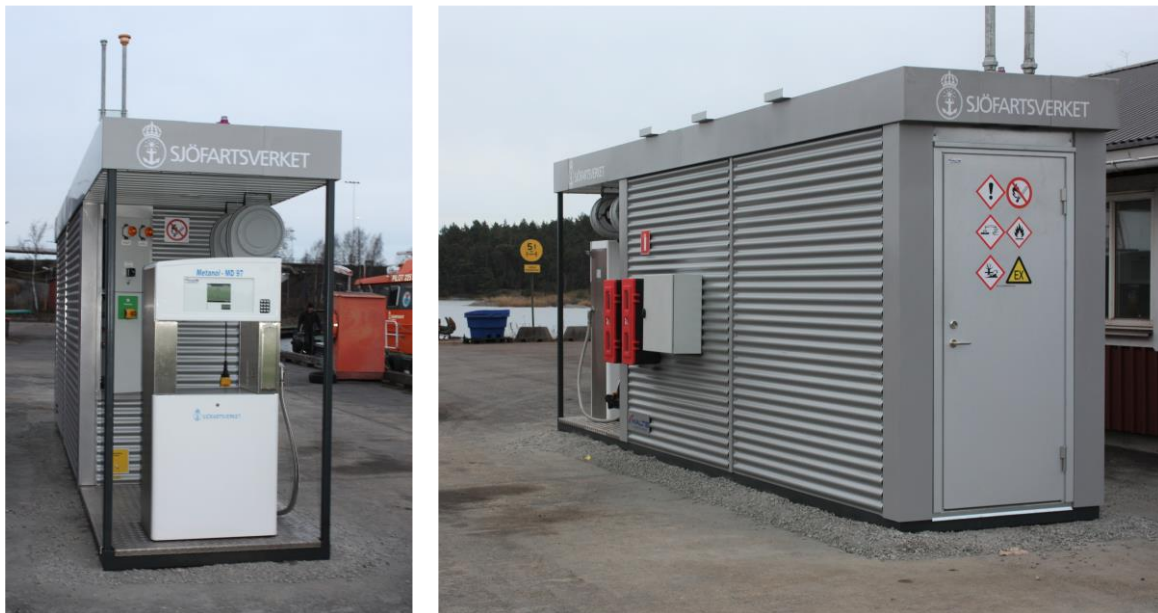
Figure 9 Methanol MD97 Fuel Dispensing Station at the Oxelösund Pilot Boat Station
