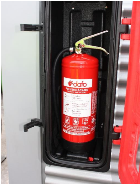
Figure 5 Dry powder based fire extinguisher suitable for methanol.
